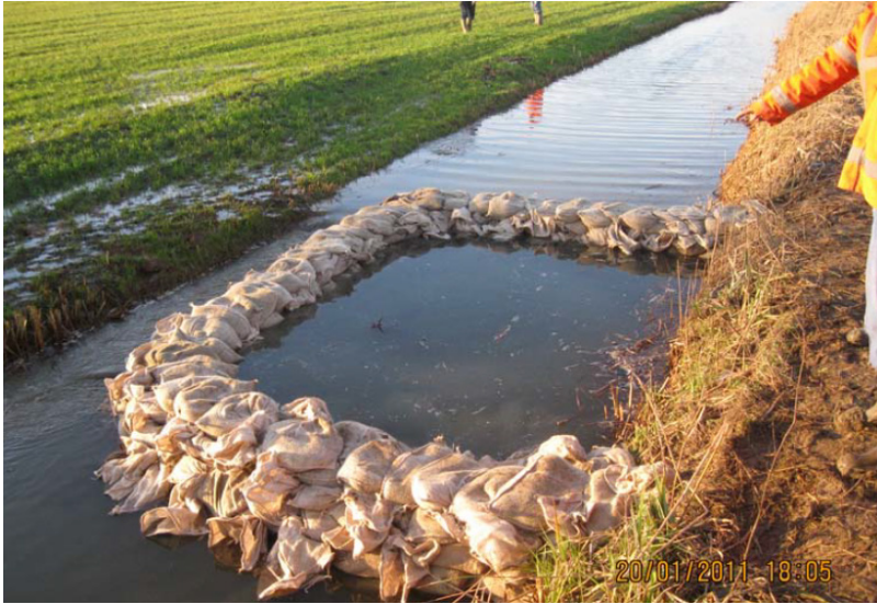
Figure 16: Sandbags to prevent piping during the high water in the year 2011 [Source: Waterschap Rivierenland]
