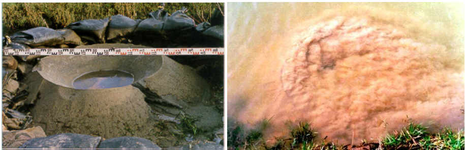
Figure 8: Sand Boils (a) post-flood, left-hand side and (b) active, right-hand side
