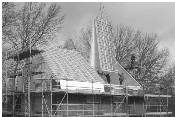
Figure 3. Structural sandwich roof element that is hoisted onto a precast concrete floor [10]
