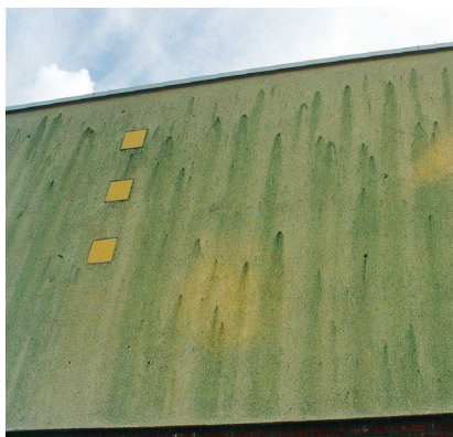
Figure 1. Fungal growth in a living room, a bathroom and algal growth on plaster
